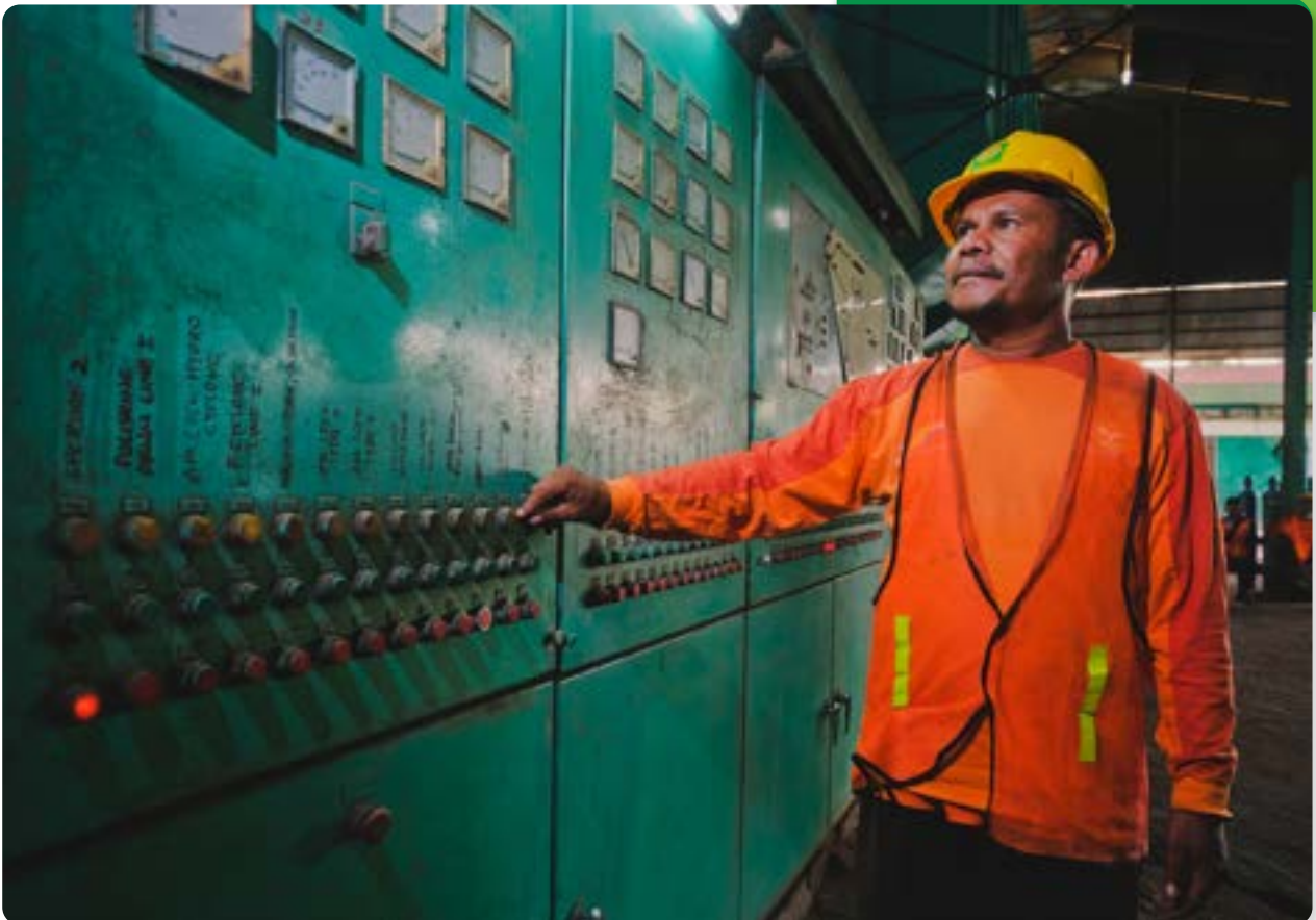
Pengawasan Panel Pabrik, Regional 8 Factory Panel Monitoring, Region 8
