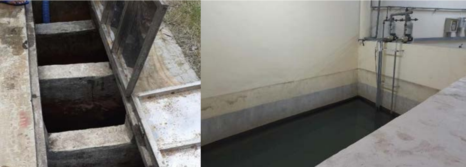
Figure 54. Canteen IPAL and Ablution Wastewater Reservoir at Jember University
