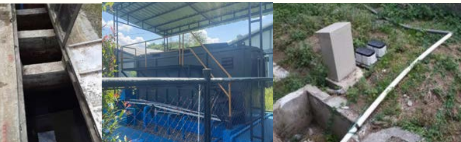
Figure 51. IPAL Canteen, Bathroom and Prayer Room
