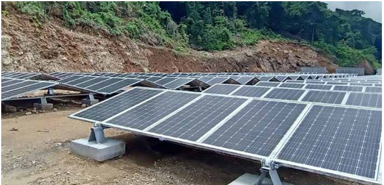
▲ Solar panel at Wetar Copper Mine
