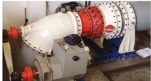
The propeller turbine at the Micro Hydro Power Plant Sengkalang with a generating power of 30 Kw. At Campus III UMM
