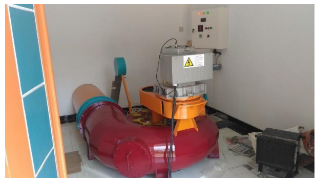
Micro Hydro Power Plant turbine house with a generating power of 10 Kw. UMM Field Laboratory - At Boon Pring
