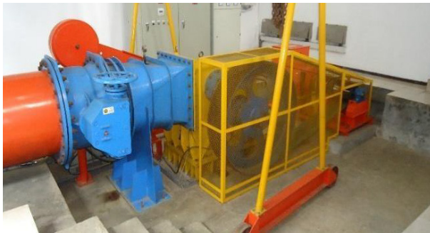
Turbine house of Micro Hydro Power Plant (PLTMH) with a generating power of 100 Kw. At Campus III UMM
