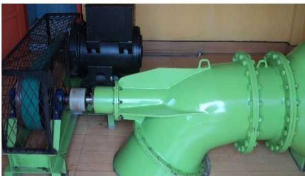
Micro Hydro Power Plant turbine house with a generating power of 45 Kw. UMM Field Laboratory - At Sumber Maron
