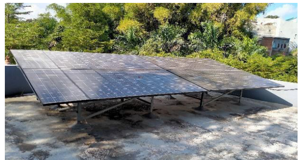
Solar Power Plant on Campus III with a power of 2500 Watt
