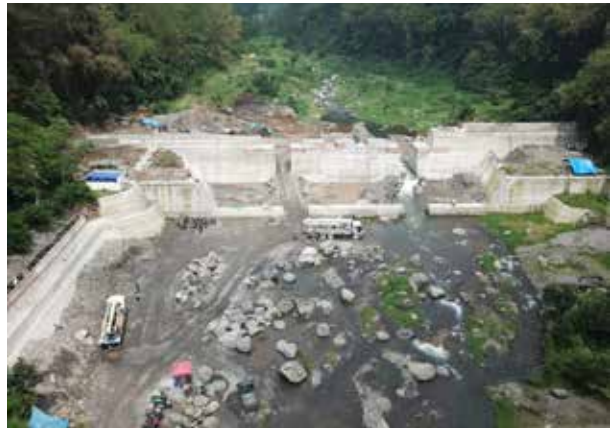
Sabo Dam Merapi
